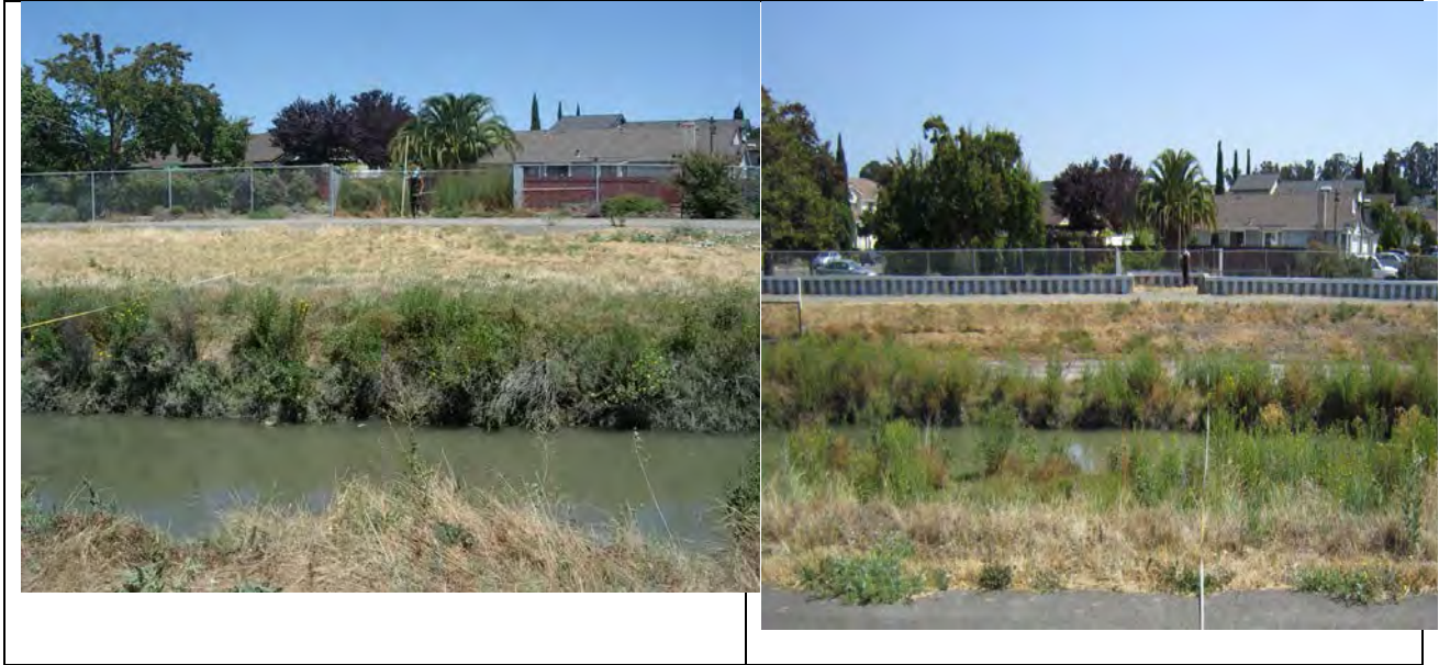
Figure 11. Channel cross section at Orleans Drive, looking at the right bank. 2009 condition on the left; 2012 condition on the right.
